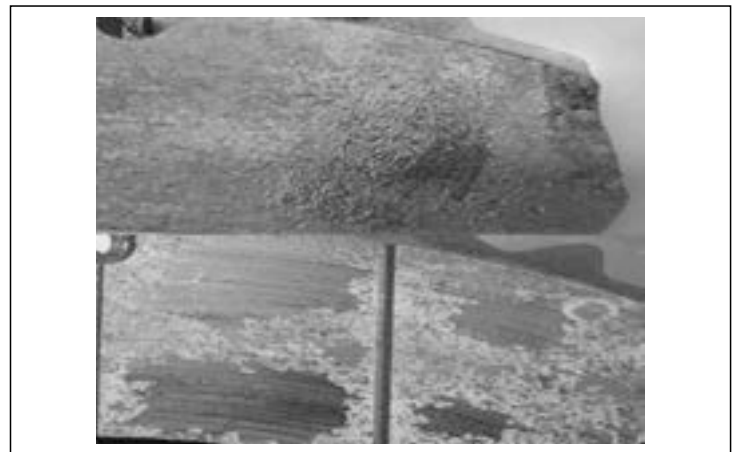
Figure13. Examples of Pads that need to be replaced
